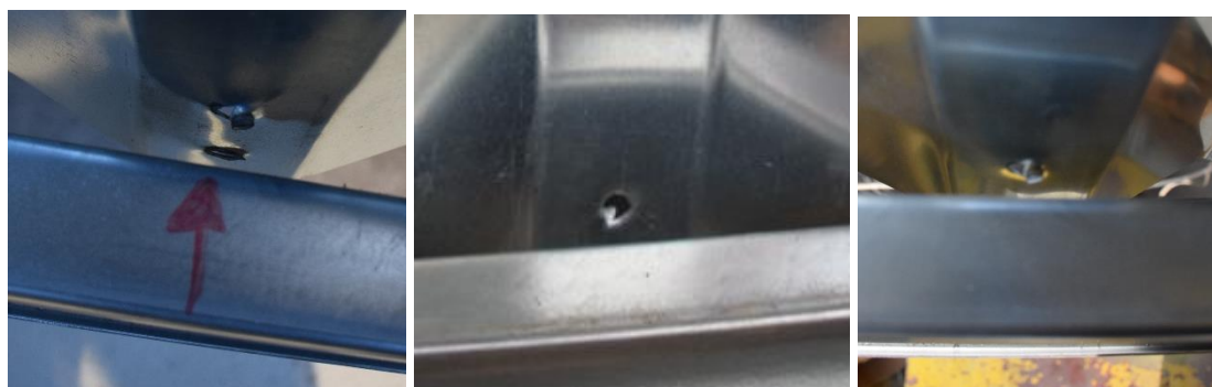
Figure 18: Spot welding failure between the web and the flange- CWB SW-1 beam.
