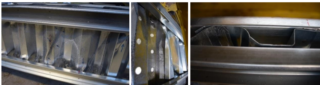
Fig. 17. Distortion of the web corrugation of the CWB SW-1 beam.
