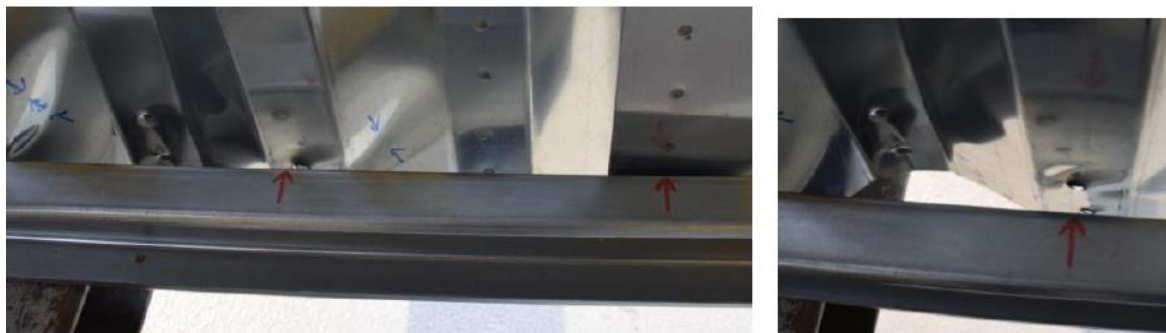
Figure 22: Spot welding failure between the web and the flange - CWB SW-2 beam.
