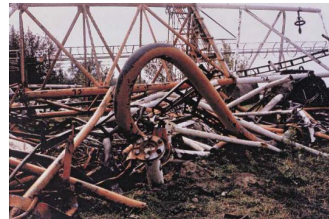
The tallest mast in the World, the 648 m high long wave mast in Konstantynow, Poland collapsed in 1991
