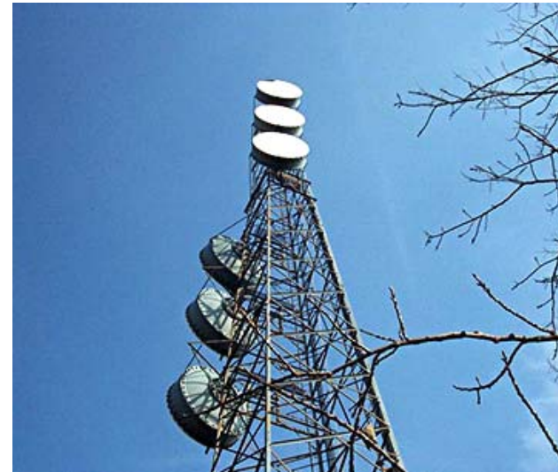
Radio Lattice Tower
