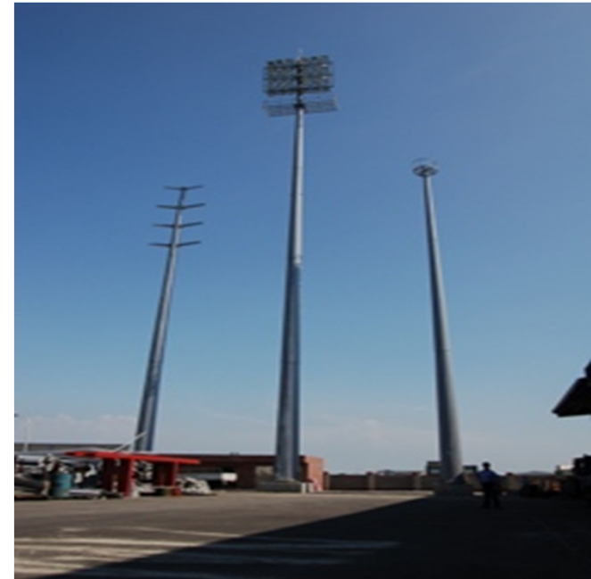
Monopoles for lighting
