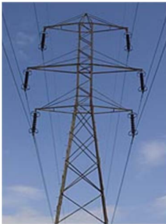
Power transmission line
