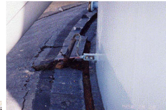
Pulled out of earthing wire
