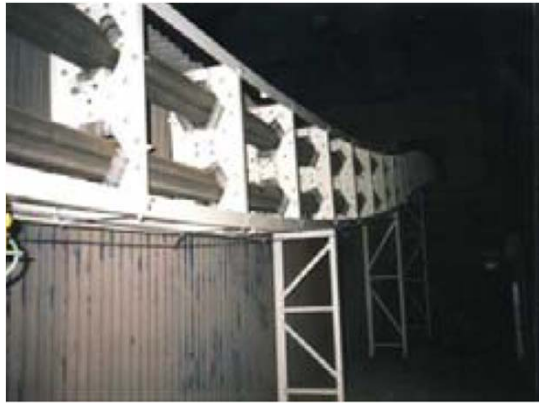
Pipelines for dusty material
