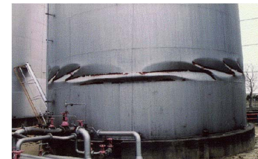
Diamond pattern buckling of tank wall
