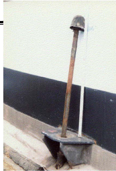
Pulled out of anchor bolt
