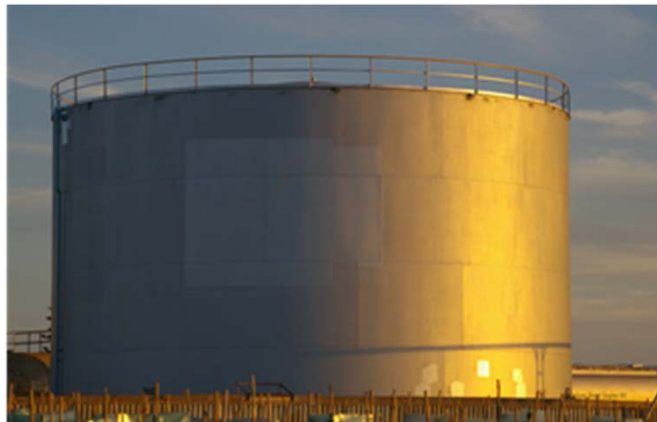
Fuel storage tank, capacity approx 2,000,000 liters, fixed roof and internal floating roof
