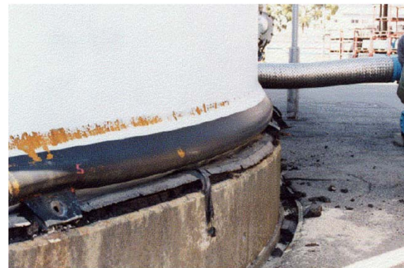
Elephant foot bulge type buckling of tank wall
