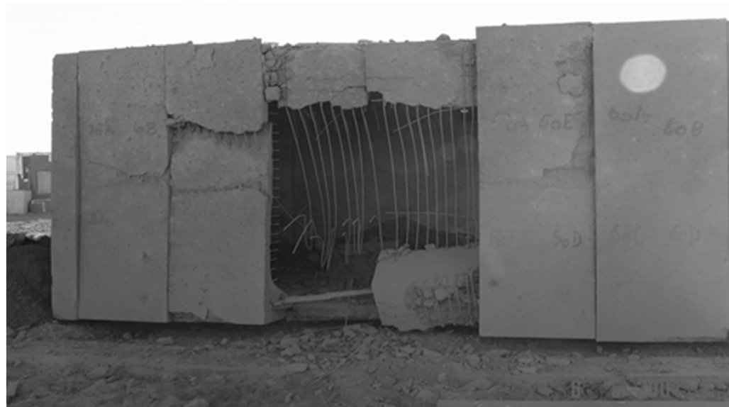
Breaching failure due to a close-in explosion of 6000kg TNT equivalent
